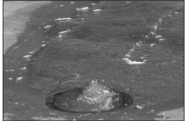
Sanitary sewer cleanout overflowing from excess grease.
